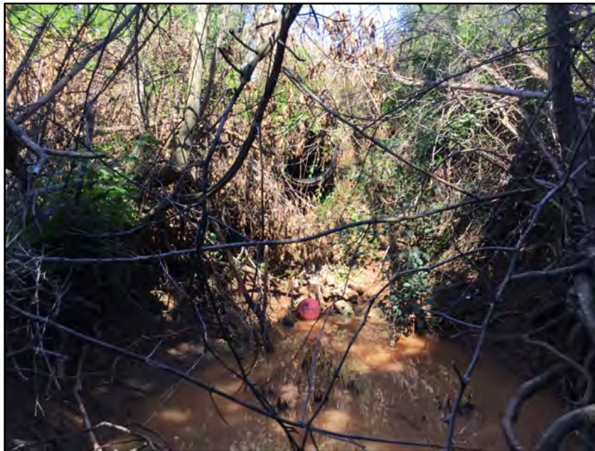
Photo 11 - View of Channel Alteration (Outlet) with Head Cutting
