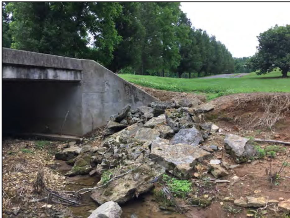
Photo 18 - View of Streambank Erosion at MS4 Outfall (Object ID 8)
