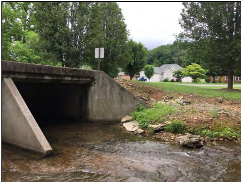
Photo 16 - View of Streambank Erosion at MS4 Outfall (Object ID 6)
