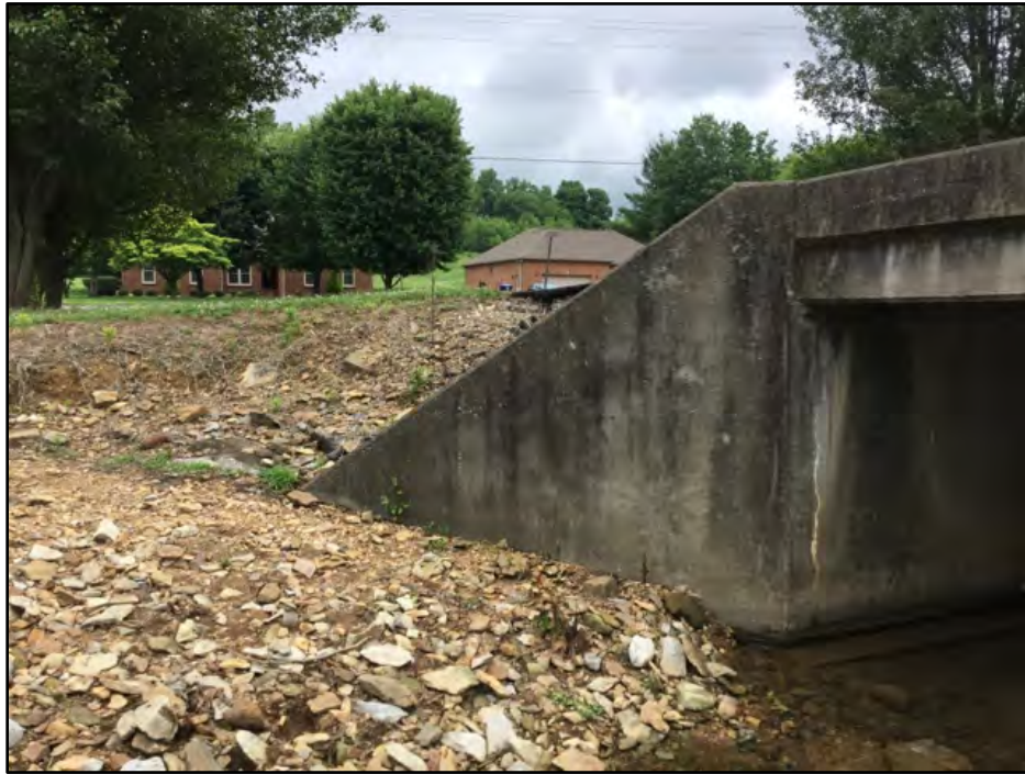
Photo 17 - View of Streambank Erosion at MS4 Outfall (Object ID 7)
