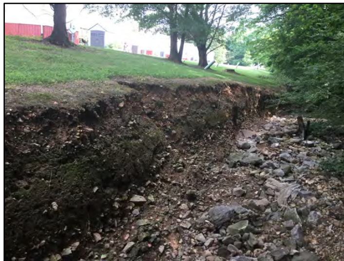
Photo 5 - View of the Erosion Site Along the Left Descending Bank
